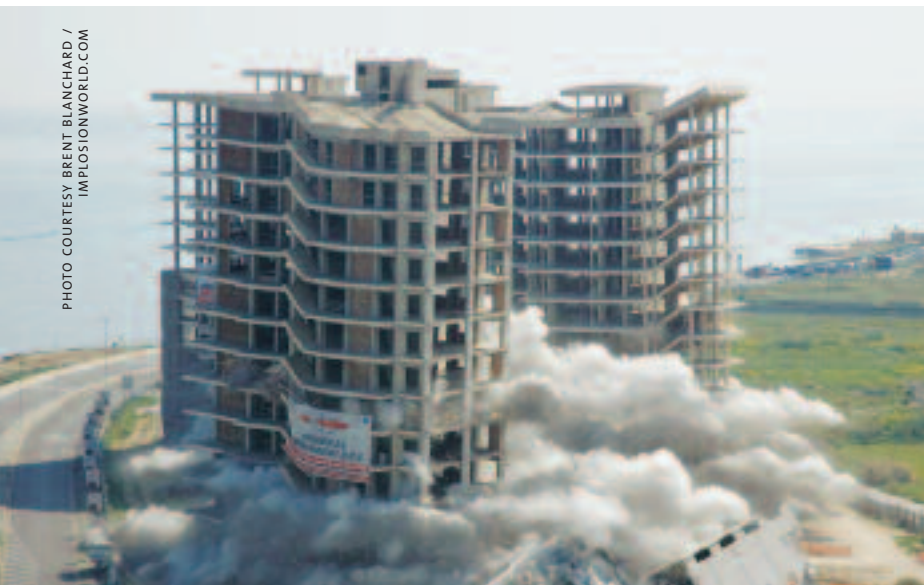
Apartments that were never completed are imploded in Bari, Italy, in 2005, below left. A worker connects detonating cord to explosives placed on a column in the Continental Bank building in Fort Worth, Texas, below right.
